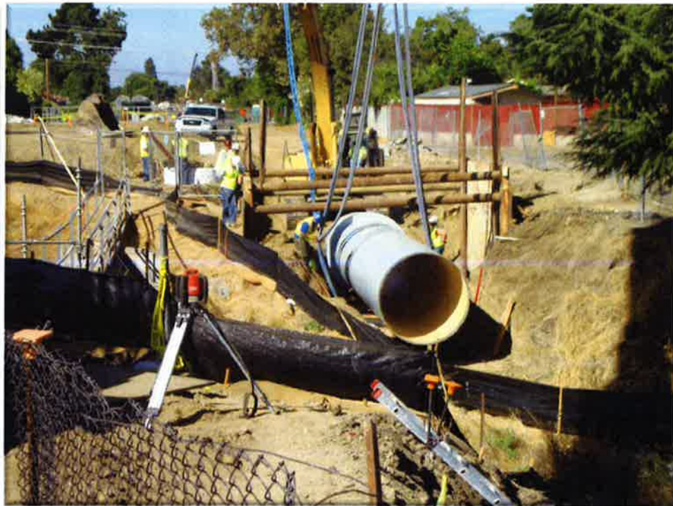
Bay Division Pipelines - # 1
