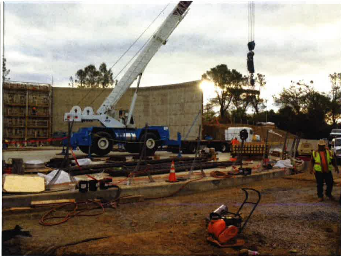
Electric Street Tank & Pipeline - # 1
