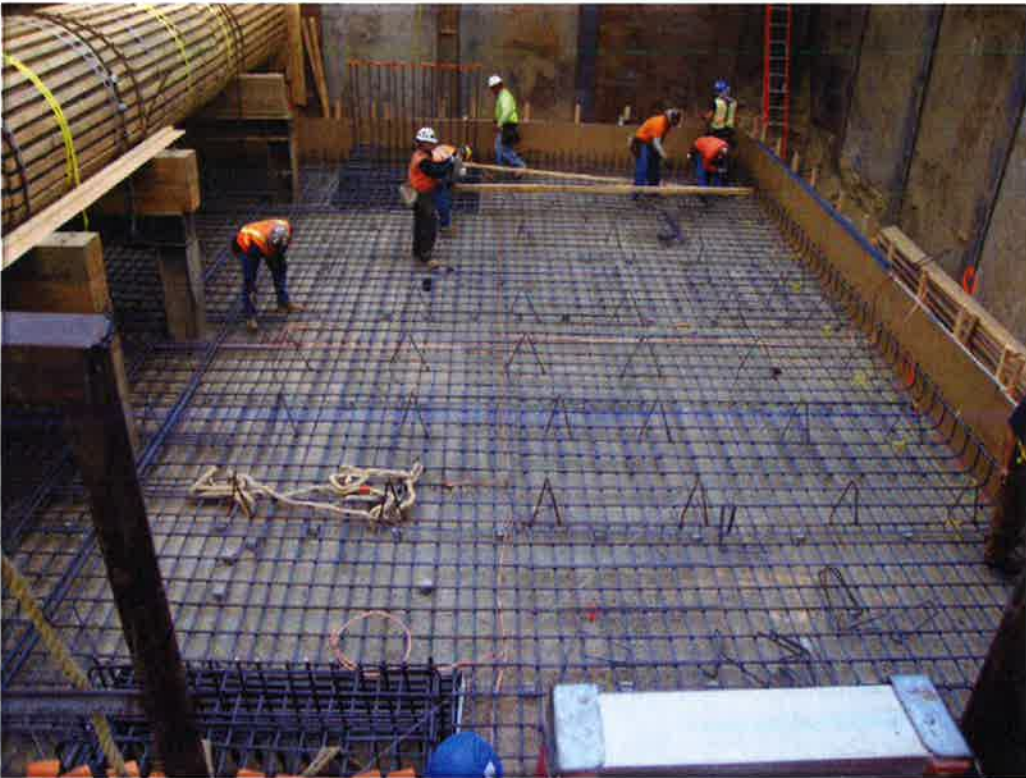
Bay Division Pipelines - # 3
