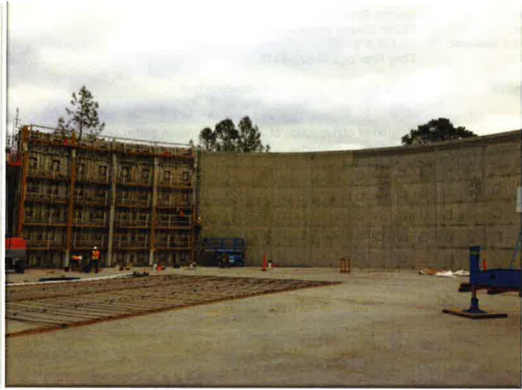
Electric Street Tank & Pipeline - # 2
